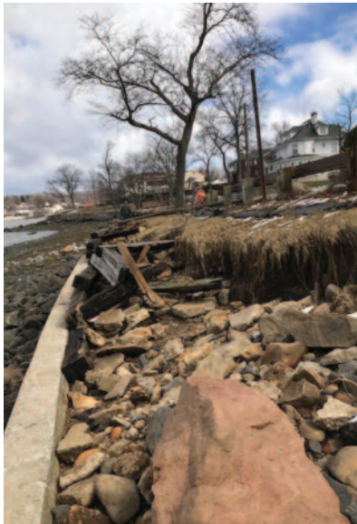
Damage at Beverley Road
