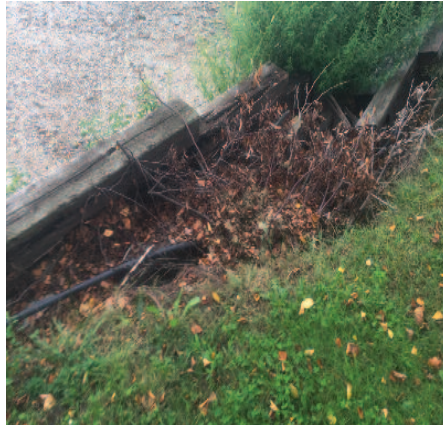
Collapse from erosion caused by scouring from storms
