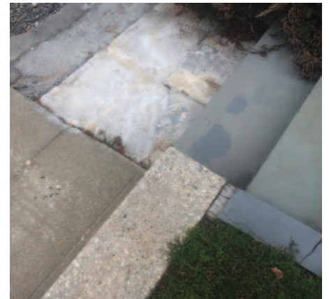
By jetty: missing bluestone and crumbling concrete - tripping hazard
