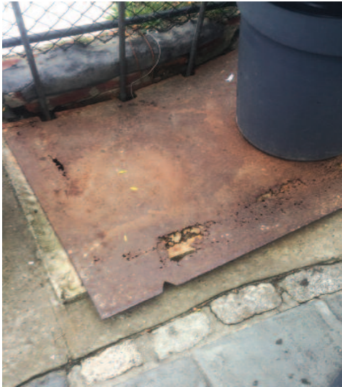
Access to plumbing behind gatehouse: metal plate is completely rusted out; needs replacement
