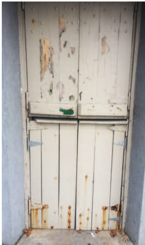
Back door of gatehouse: cracked glass and metal trim rusting & pulling away from door frame. Front door of gatehouse: no words needed.
